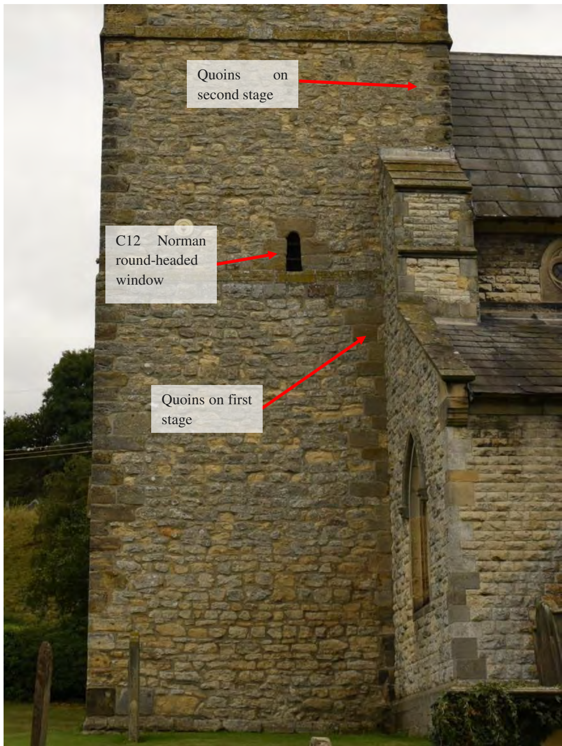
Figure 113: The first two stages of the tower exhibit matching quoining and coursed rubble masonry, and are therefore contemporaneous, but the quoining on each stage of the eastern wall does not align, indicating that the second stage was built over an earlier nave wall. The Norman round-headed window in the second stage is also shown (Source: Author 2019).
