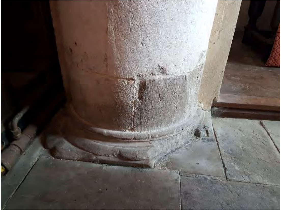
Figure 32: The base of the eastern column of the eastern bay of the southern arcade (Source: Author 2019).
