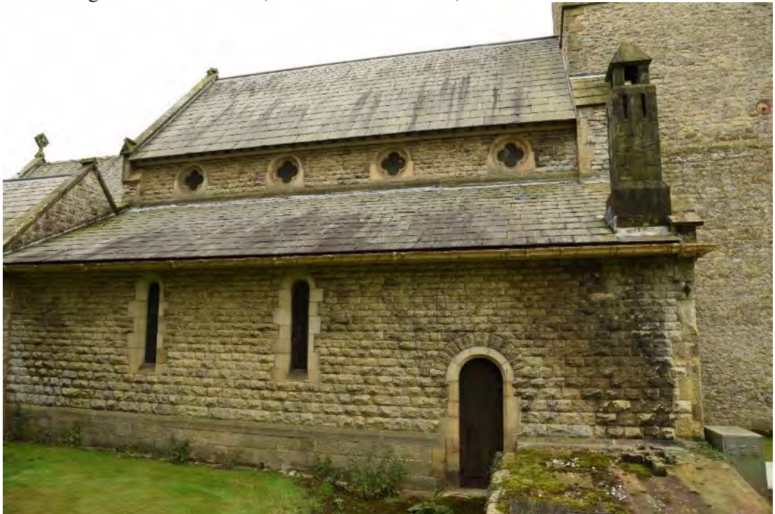
Figure 74: The northern elevation of the three bays of the north aisle, showing the Victorian Norman style door and lancet windows, with the four-bayed clerestory above (Source: Author 2019).
