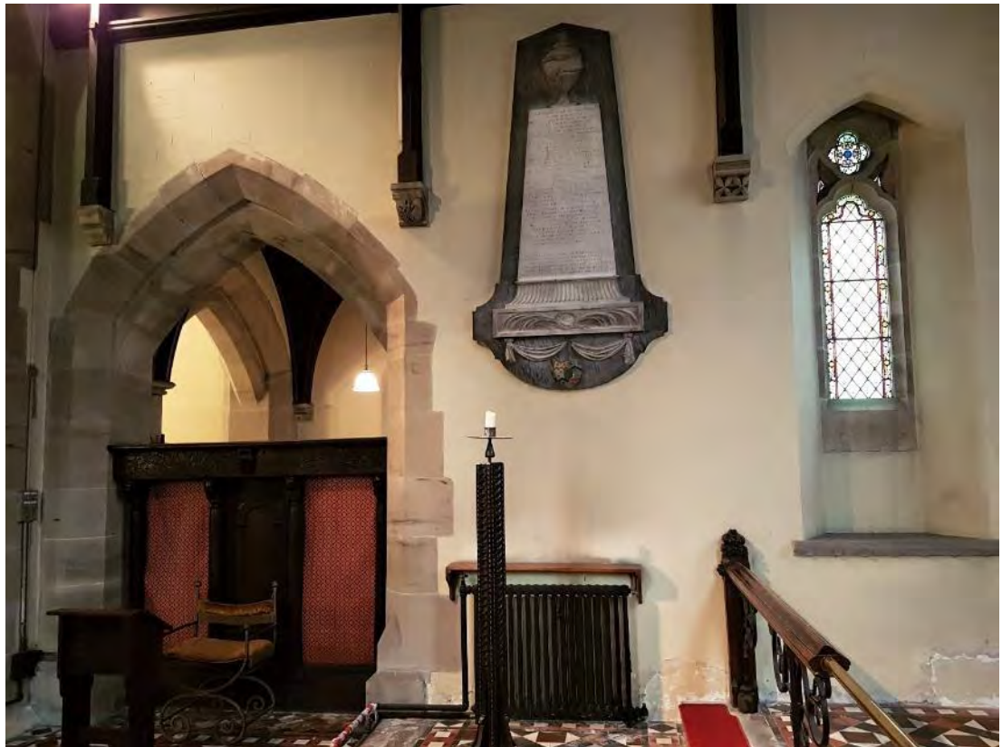
Figure 95: The northern interior wall of the chancel, showing the scored plasterwork, as well as the double-chamfered arch into the vestry in the eastern bay, the eighteenth-century memorial to members of the Comber family in the central bay, and the one-light Victorian Middle Decorated Gothic window in the eastern bay (Source: Author 2019).
