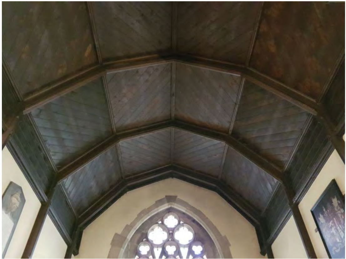
Figure 106: The Victorian gabled gambrel ceiling with diagonally set timber boards, supported by four geometric gambrel trusses on a mix of floriolate, geometric and crested corbels (Source: Author 2019).
