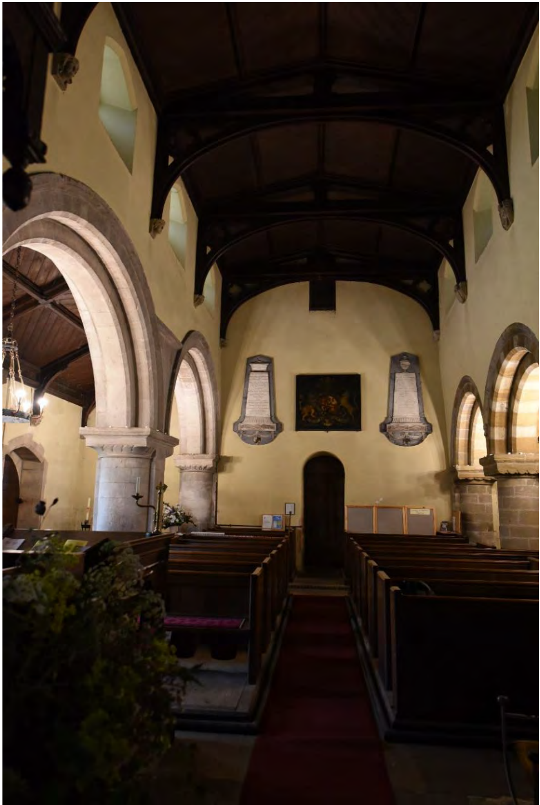
Figure 39: The roof of the nave, showing timber beams resting on corbels, supporting a timber-boarded low-pitched ceiling (Source: Author 2019).
