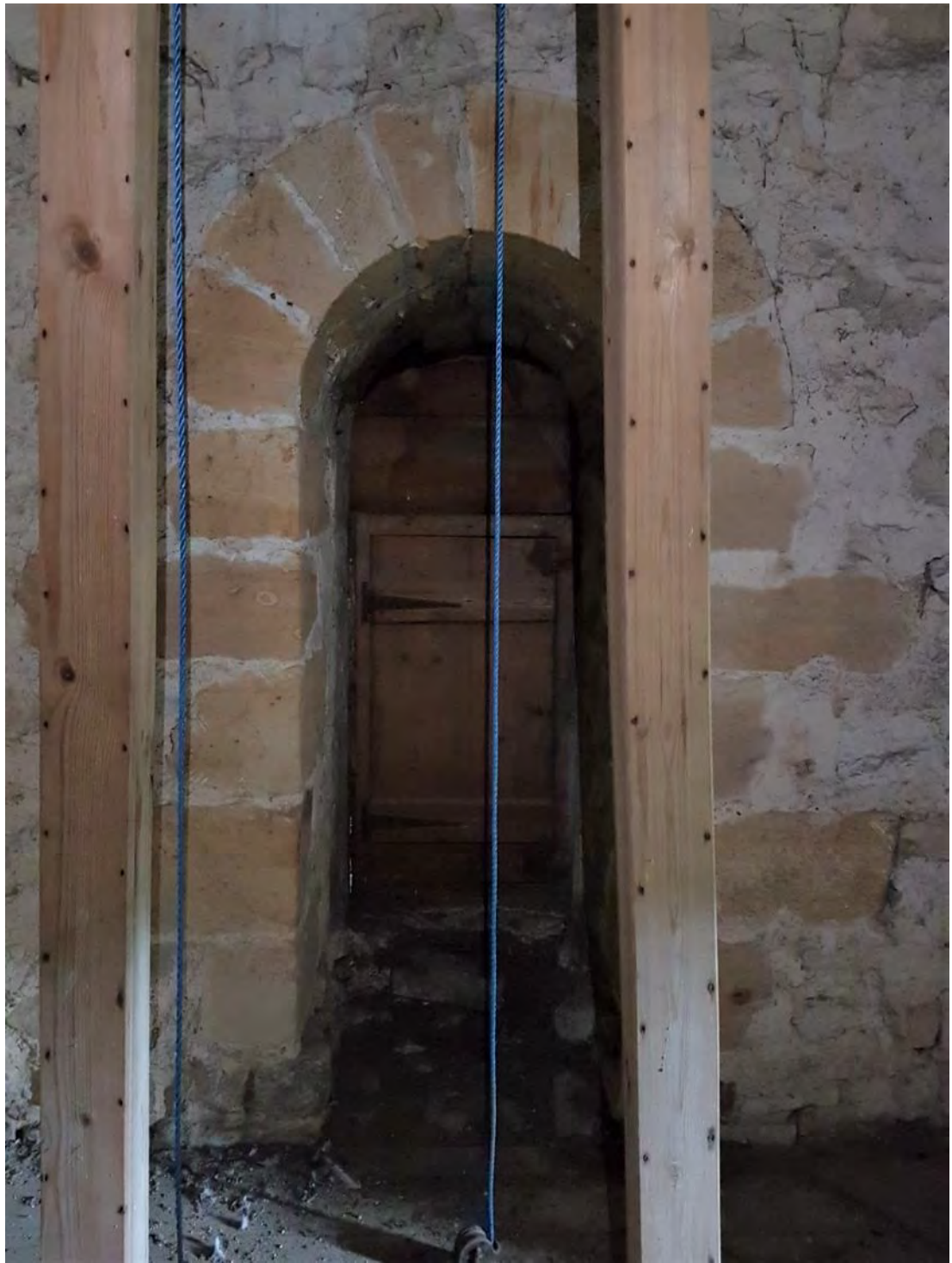
Figure 132: The twelfth-century Norman round-headed door in the eastern wall of the tower, showing the inserted timber door, with the timbers supporting the belfry above in the foreground (Source: Author 2019).
