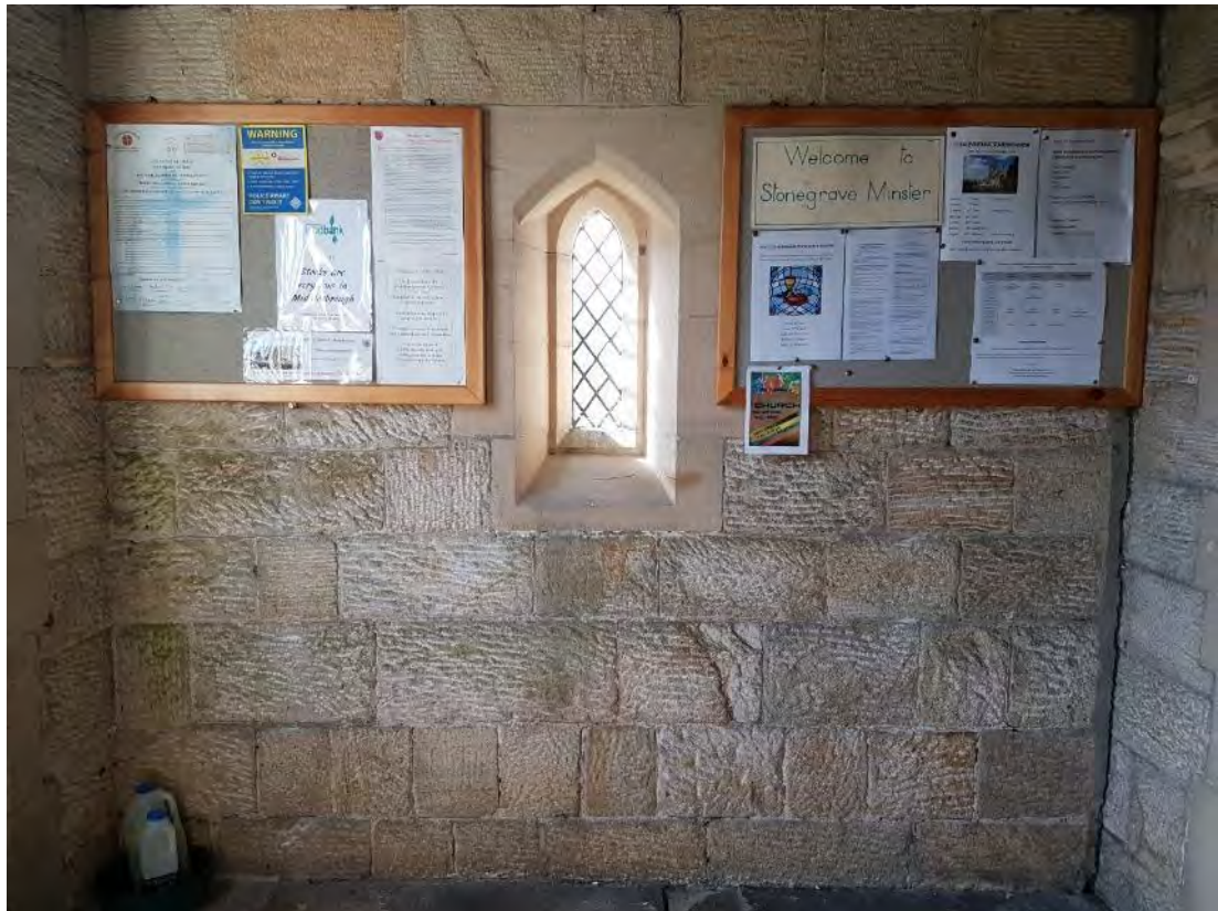
Figure 69: The western internal elevation of the porch, showing the mixed tooling marks and mix of soldier and Flemish bonding, which is unusual for stonework. The interior of the lancet window can also be seen, displaying a segmental pointed arch on the interior face and a chamfered surround. The tooling on the stone coursing is coarse and irregular, with a mix of orientations, but mostly horizontal (Source: Author 2019).
