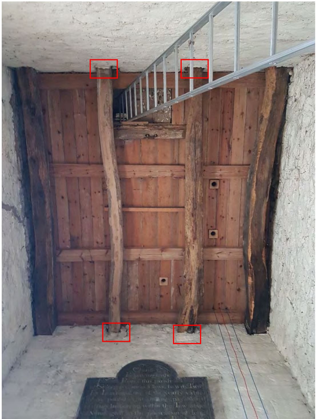
Figure 196: The exposed ceiling of the first stage of the tower, showing the built-up areas of stonework around the central beams outlined in red (Source: Author 2019).
