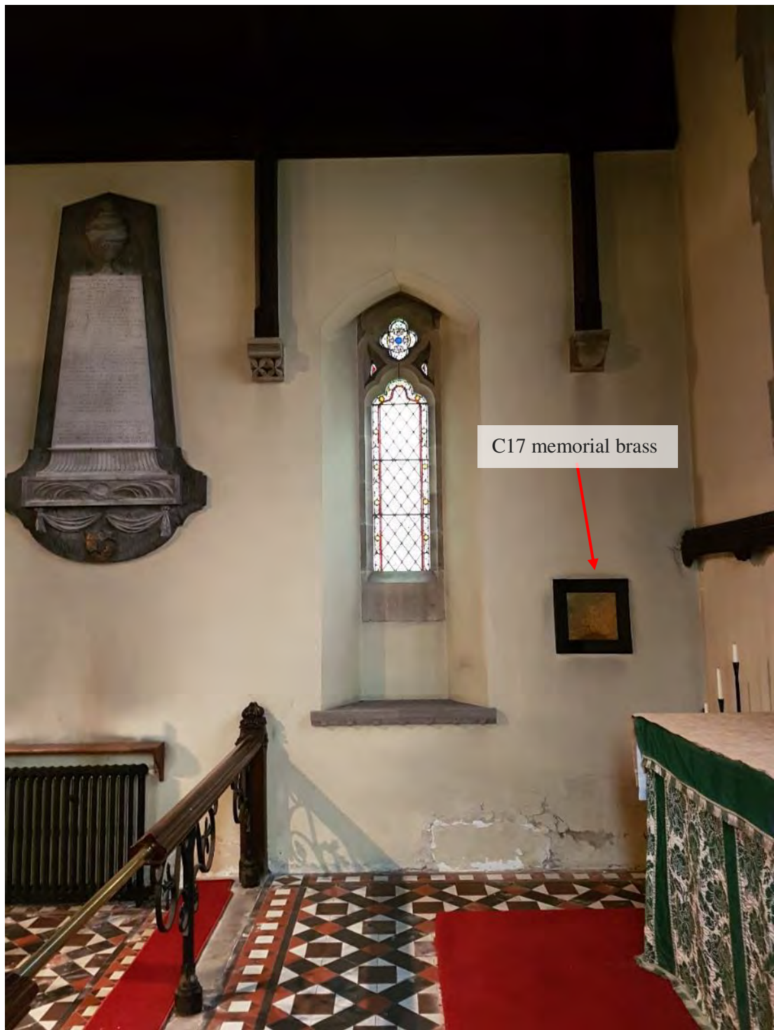
Figure 103: The northern wall of the eastern bay of the chancel, showing the location of the seventeenth-century memorial brass to Dean Thomas Comber's wife, Alice (d. 1720) and their son, William (d. 1702), re-mounted on black marble during the Victorian restoration (Source: Author 2019).
