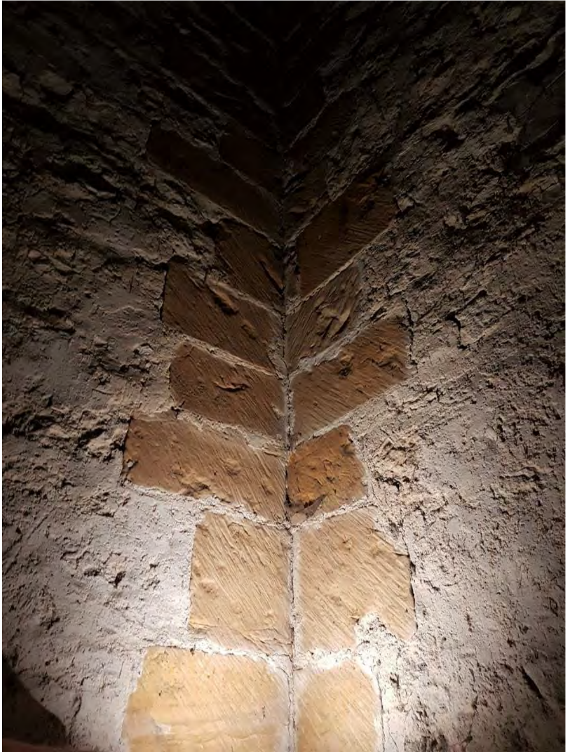
Figure 130: The oblique twelfth-century tooling of the quoining in the second stage of the tower (Source: Author 2019).
