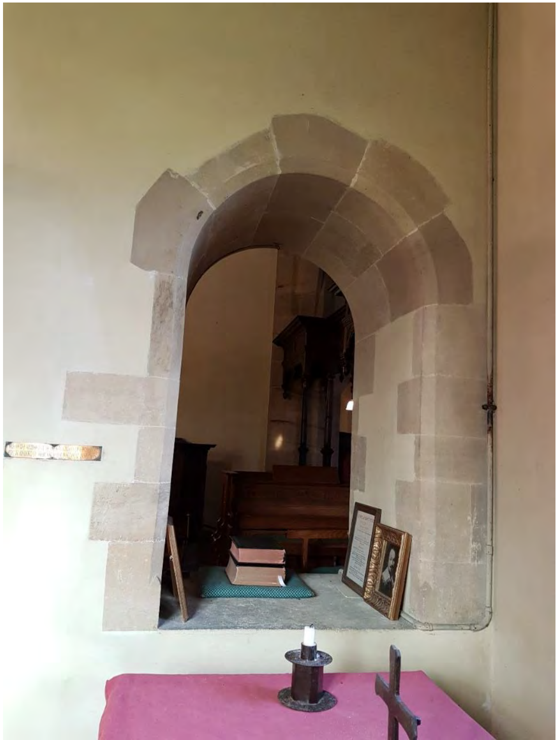
Figure 54: The opening in the eastern chapel, with the nave in the background (Source: Author 2019).
