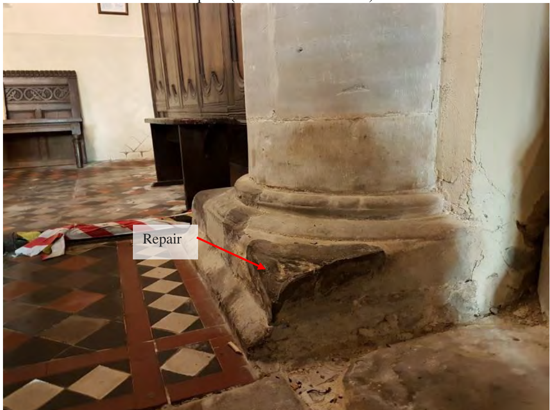
Figure 152: The eastern end of the northern arcade, showing the cementitious repair to the base of the eastern column, which may be evidence of the location of the three-decker pulpit (Source: Author 2019).
