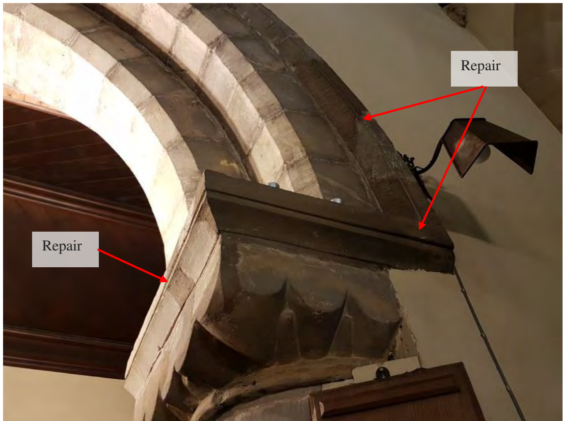
Figure 151: The eastern end of the northern arcade, showing the cementitious repair to the chamfered label and the capital (Source: Author 2019).
