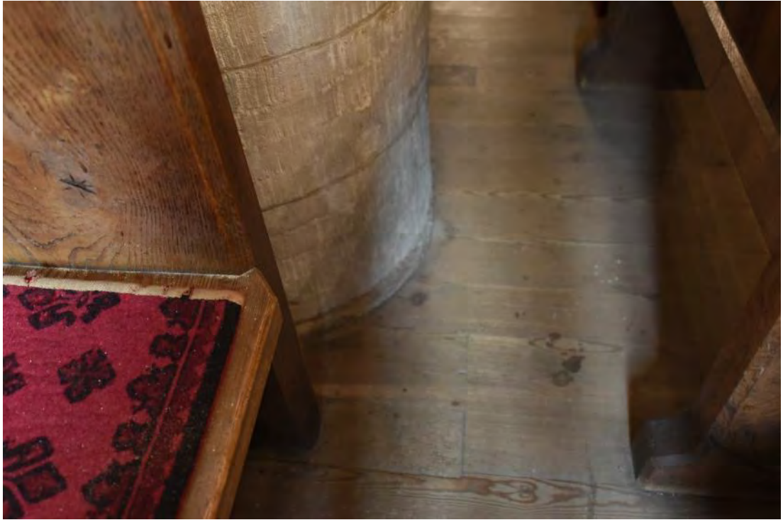
Figure 34: The base of the western column of the eastern bay of the southern arcade (Source: Author 2019).
