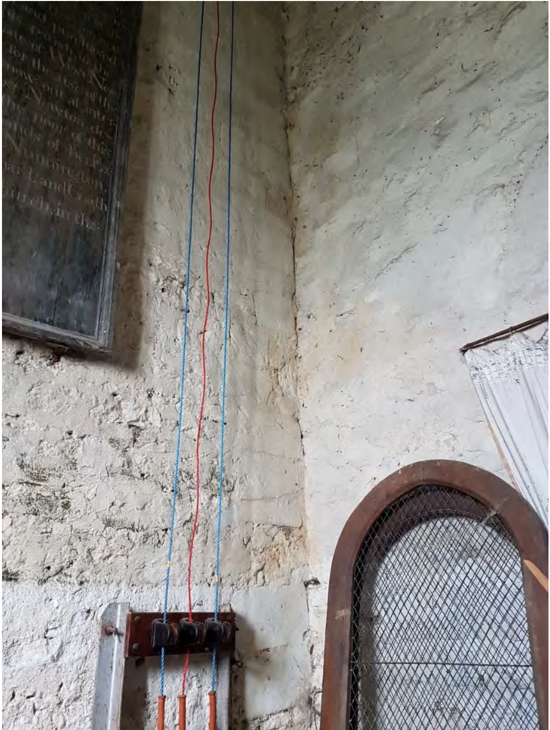
Figure 120: The interior of the first stage of the tower, looking north-east to the straight joint between the northern and eastern walls of the tower, showing that the north walls abuts the east wall (Source: Author 2019).
