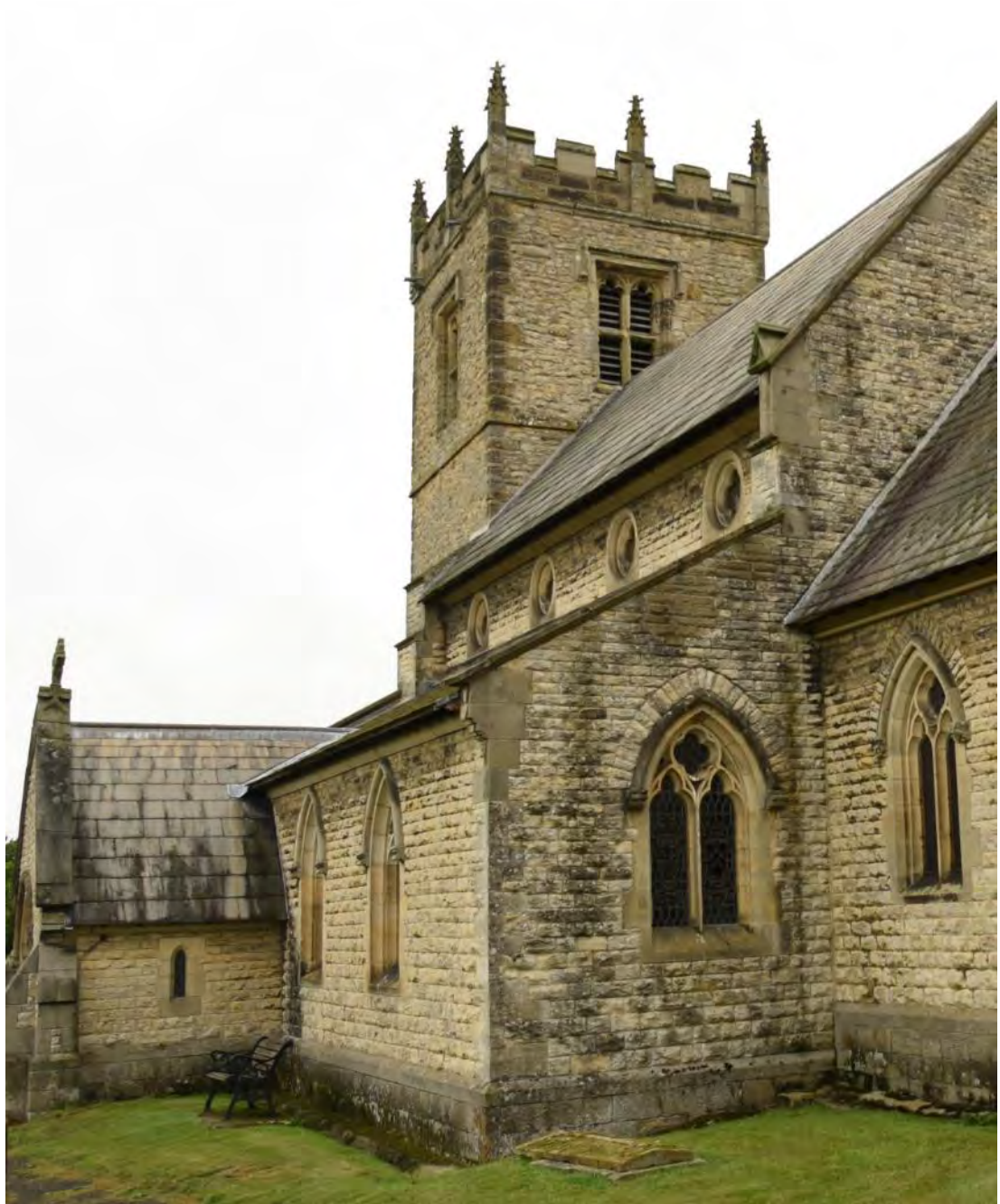
Figure 112: The eastern elevation of the three-stage square tower, constructed from coursed rough limestone rubble with dressed calcareous sandstone quoining, showing the fifteenth-century Perpendicular belfry (Source: Author 2019).
