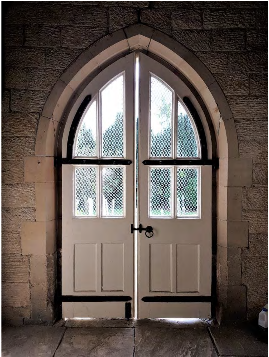
Figure 70: The southern internal elevation of the porch, showing the rear of the front pointed-arch door, displaying a chamfered arch with a chamfered quoin surround with a pyramid stop at the base of the surround. The tooling on the stone coursing is coarse and irregular, with a mix of orientations, but mostly horizontal (Source: Author 2019).
