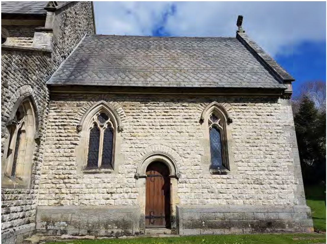
Figure 91: The southern elevation of the chancel, showing the cusped two-light Victorian Middle Decorated Geometric Gothic pointed arch window with quatrefoil tracery in the western bay, the Victorian Norman style door in the central bay and the a trefoil-headed one-light Victorian Middle Decorated Geometric Gothic pointed arch window with quatrefoil tracery in the eastern bay (Source: Author 2019).
