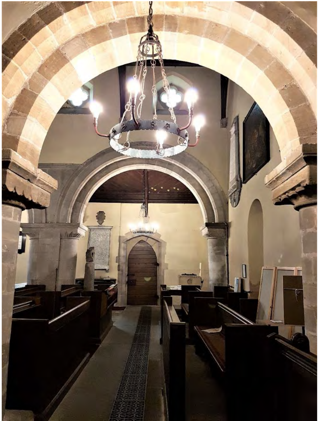
Figure 44: The line of the underfloor heating and ventilation surrounded by 1862-3 floor slabs, taken from the north (Source: Author 2019).
