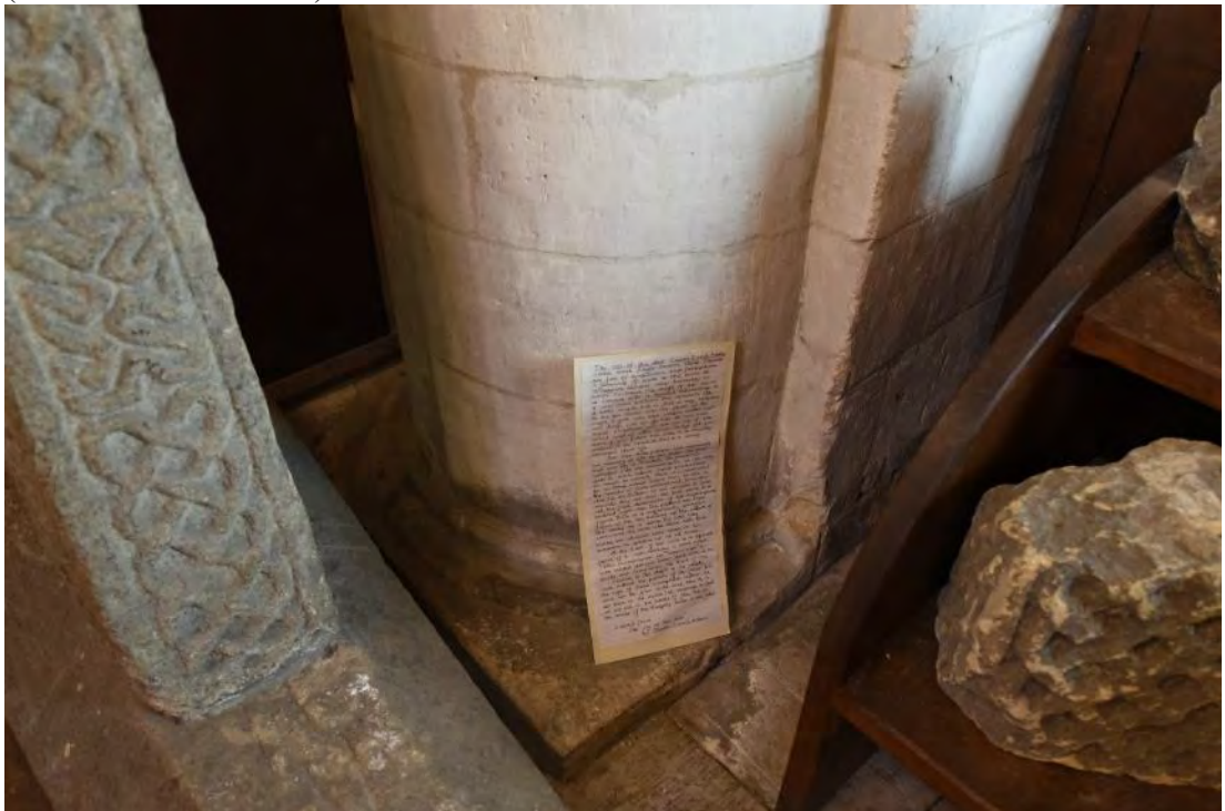
Figure 33: The base of the eastern column of the western bay of the southern arcade (Source: Author 2019).
