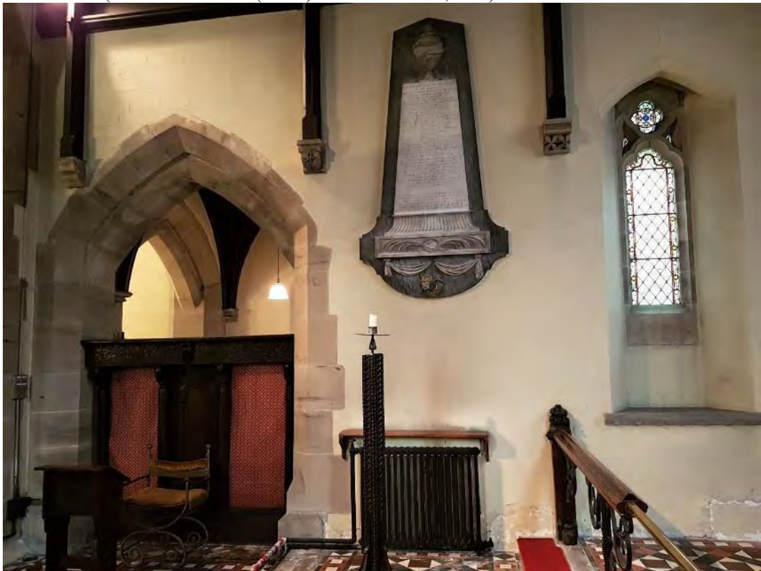
Figure 176: The existing north chancel wall, showing the extant arch into the chancel bay of the north aisle (Source: Author 2019).
