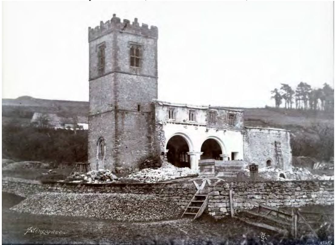
Figure 15: Photograph by George Fowler Jones during the 1862-3 restoration, showing the exterior of the church from the south-west. It shows the demolition of the southern aisle and evidence of the previous roofing in of the western end of the clerestory (Source: NSM RPS 18951).
