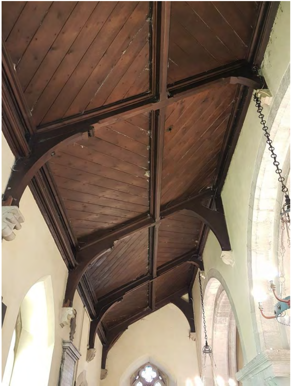
Figure 62: The roof of the south aisle, showing the 1862-3 timber trusses resting on 1862-3 corbels, with diagonal timber boards, looking west (Source: Author 2019).
