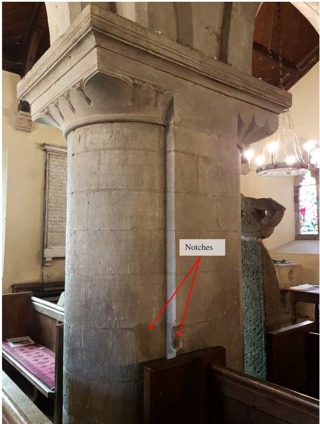
Figure 156: The central pillar of the southern arcade, showing the repaired notches, possibly a result of the installation of the box pews (Source: Author 2019).
