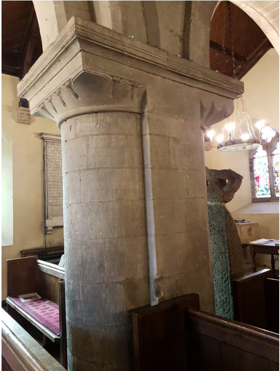
Figure 30: The central pier between the western and eastern bays of the southern arcade, showing the scalloped trumpet capital with nailhead decoration on the western column and waterleaf capitals on the eastern capital (Source: Author 2019).
