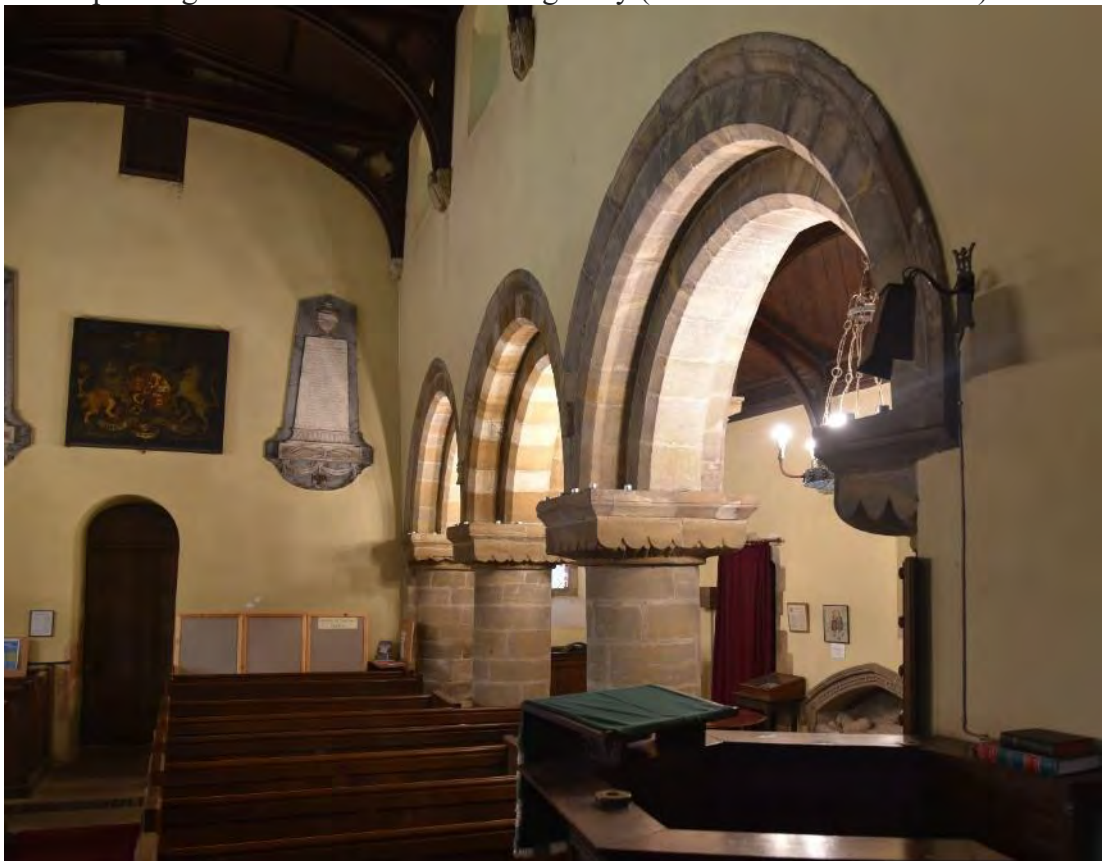
Figure 145: Photograph taken in 2019, showing the interior, demonstrating the plastered walls and the repair work to the arcade (Source: Author 2019).
