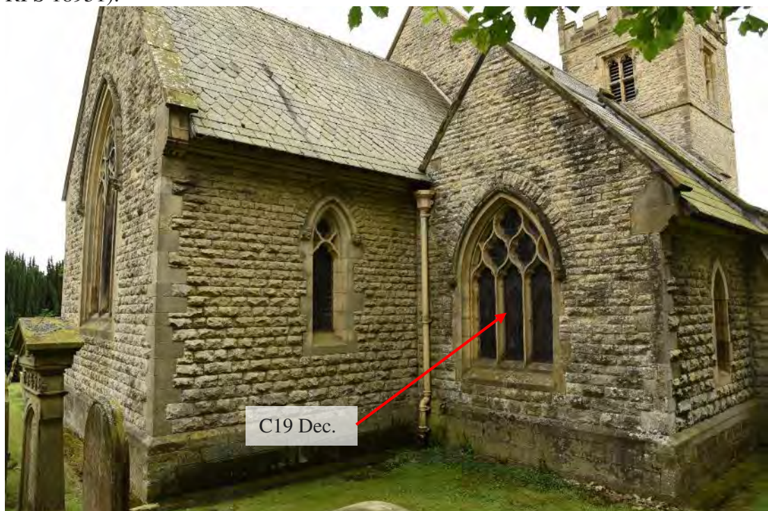
Figure 168: The existing eastern elevation of the northern aisle, showing the extant Victorian reproduction of the earlier C14 three-light Decorated Gothic window (Source: Author 2019).
