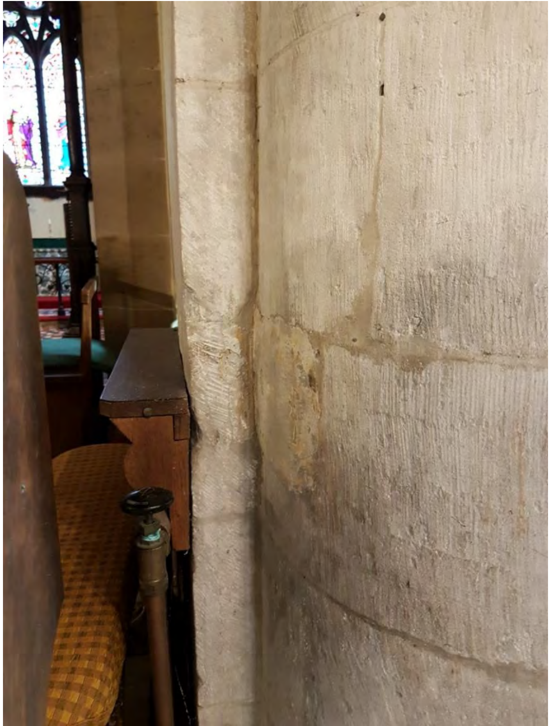
Figure 154: Repair from fixing of box pews to eastern column of southern arcade (Source: Author 2019).
